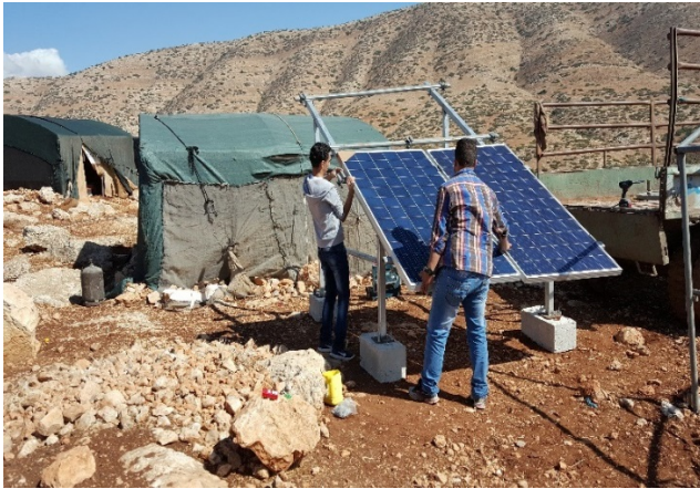
Figure 4: This photo was taken during the installation of solar units in Al Maleh Community
